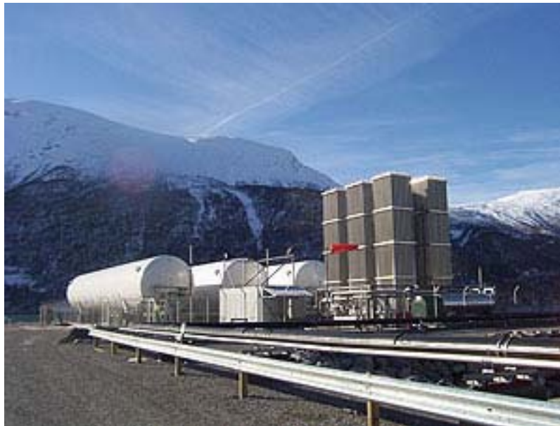
Figure 2-4 LNG receiving and storage terminal (Source: MARINTEK)
