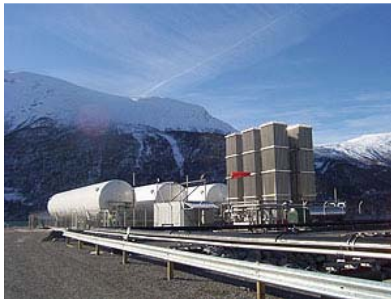
Figure 11-3 LNG receiving and storage terminal (Source: MARINTEK)
